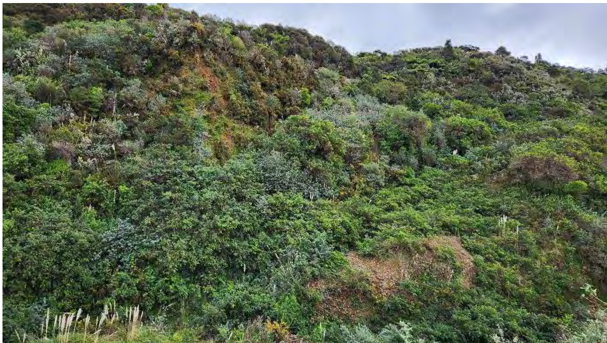
Figure 4-5: Examples of localised rock fall in former quarry batters
