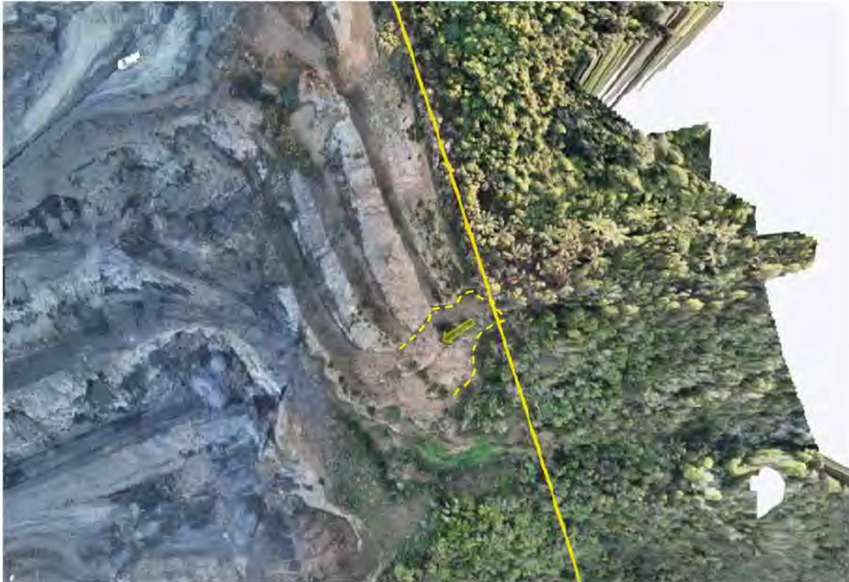
Figure 5-5: Existing instability in Area C. Belmont East wall abutting the Firth Block.
