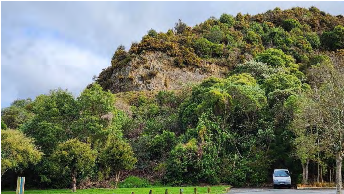
Figure 4-6: Unsupported cut slopes within Belmont Regional Park
