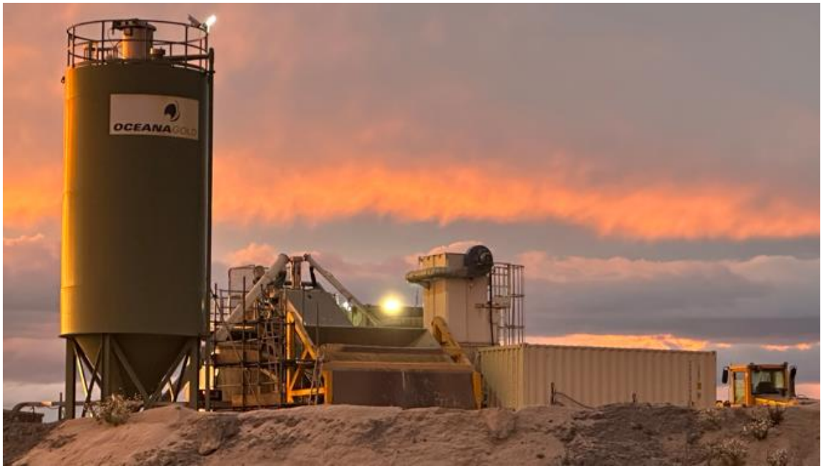
B2.9: Concrete Batching Plant (Structure mounted lights)
