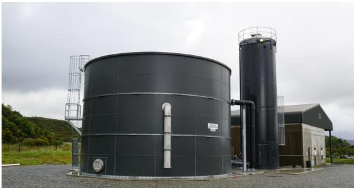
Figure 6. Water Treatment Plant – Similar Installation (Courtesy of Process Flow)
