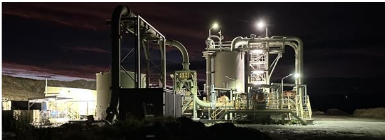
B5.6: Pump Station
