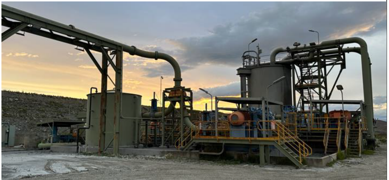
B2.1: Pump Station (Column & structure mounted lights)
