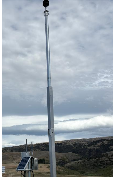
Figure 12: Photograph of the Lake Clearview meteorological monitoring equipment
