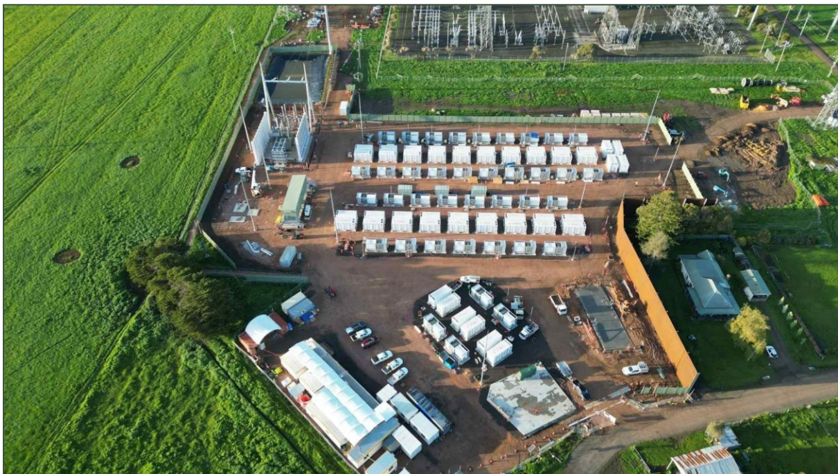
Figure 7: Representative example of a BESS next to a substation
