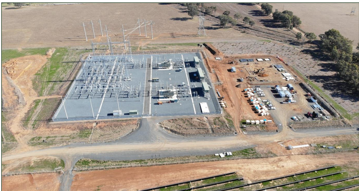
Figure 6: Example of a new substation for a solar farm connection (Walla Walla Substation, Australia)
