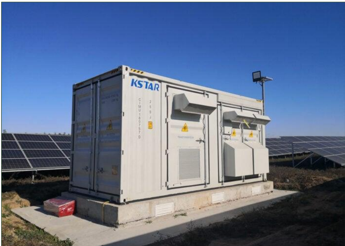
Figure 3: Representative example of a central inverter unit
