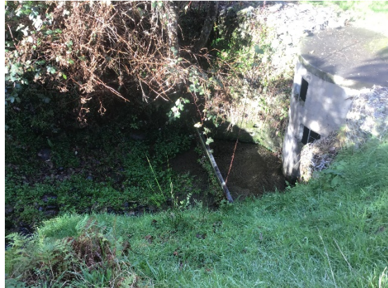
Photo 11: Manhole/riser at the downstream extent of Stream A
