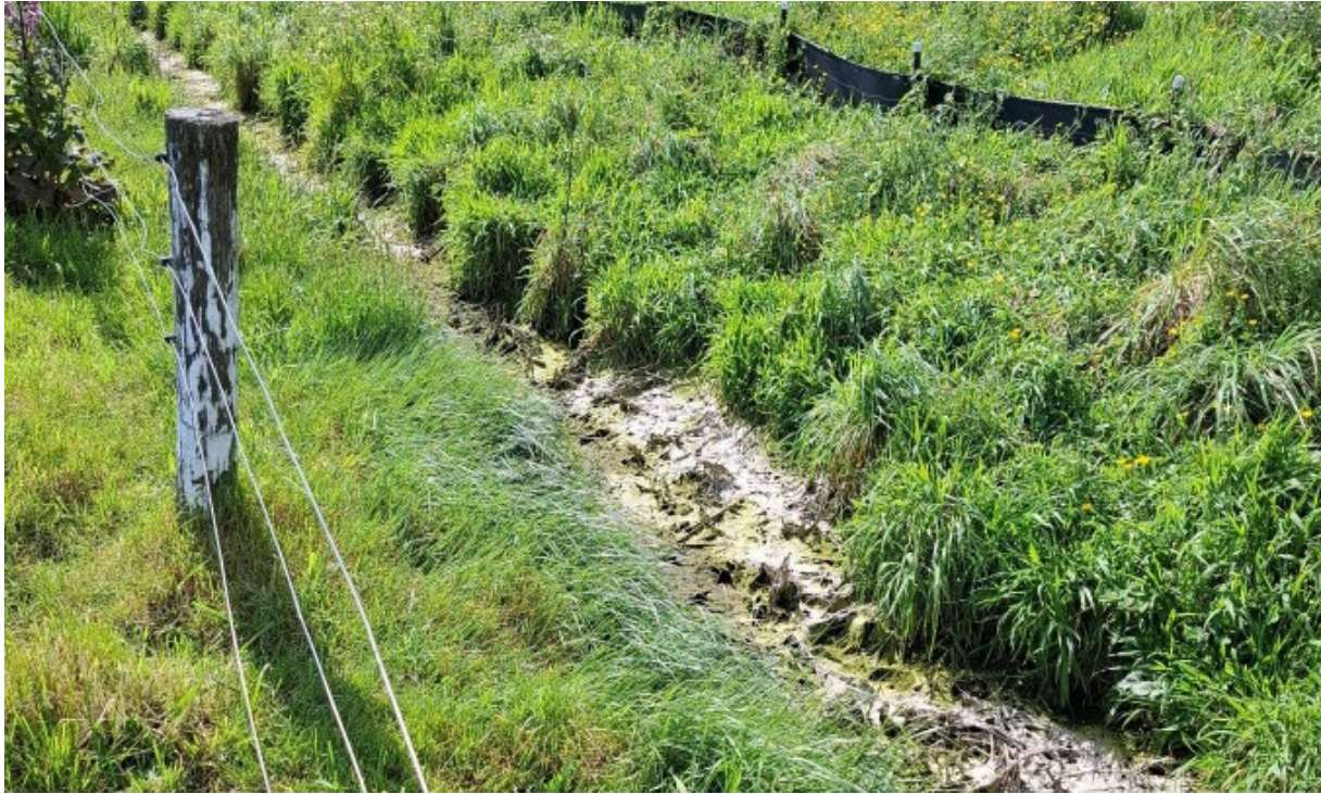
Figure 14. Drain condition example (ecoLogical Solutions).
