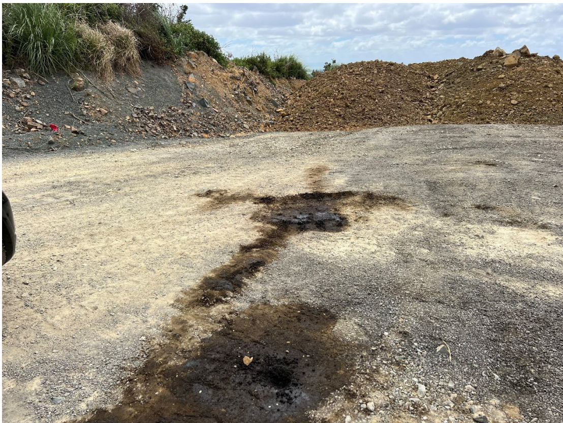
Photograph 6: Overview of the western portion of the Graveyard area where fresh hydrocarbon staining was observed and PMS10 was collected. The stockpile of material (assumed overburden) that was observed to be dumped by a truck during the site walkover is in the background.
