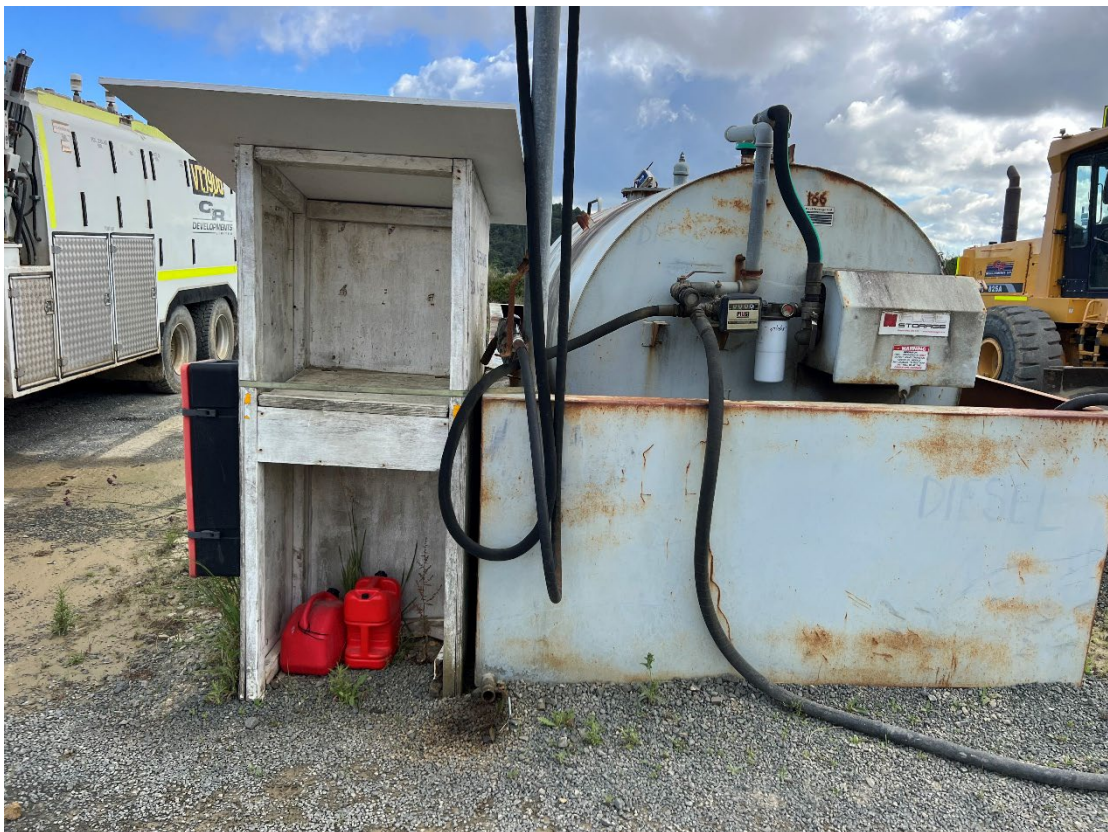
Photograph 10: Looking northeast at the eastern AST with hydrocarbon staining on the ground where PMS12 was taken.
