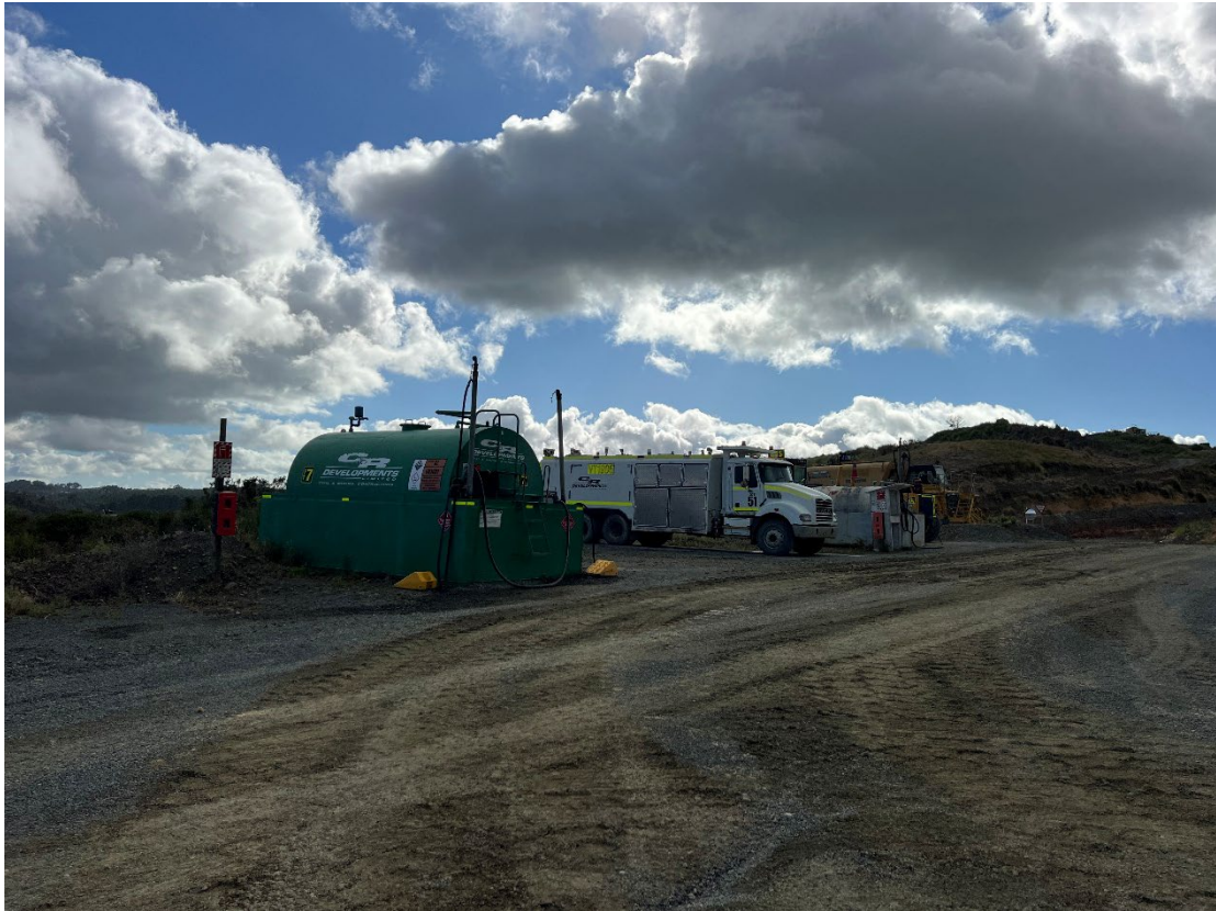
Photograph 9: Looking northeast at 2x bunded ASTs located in the C+R Rack.
