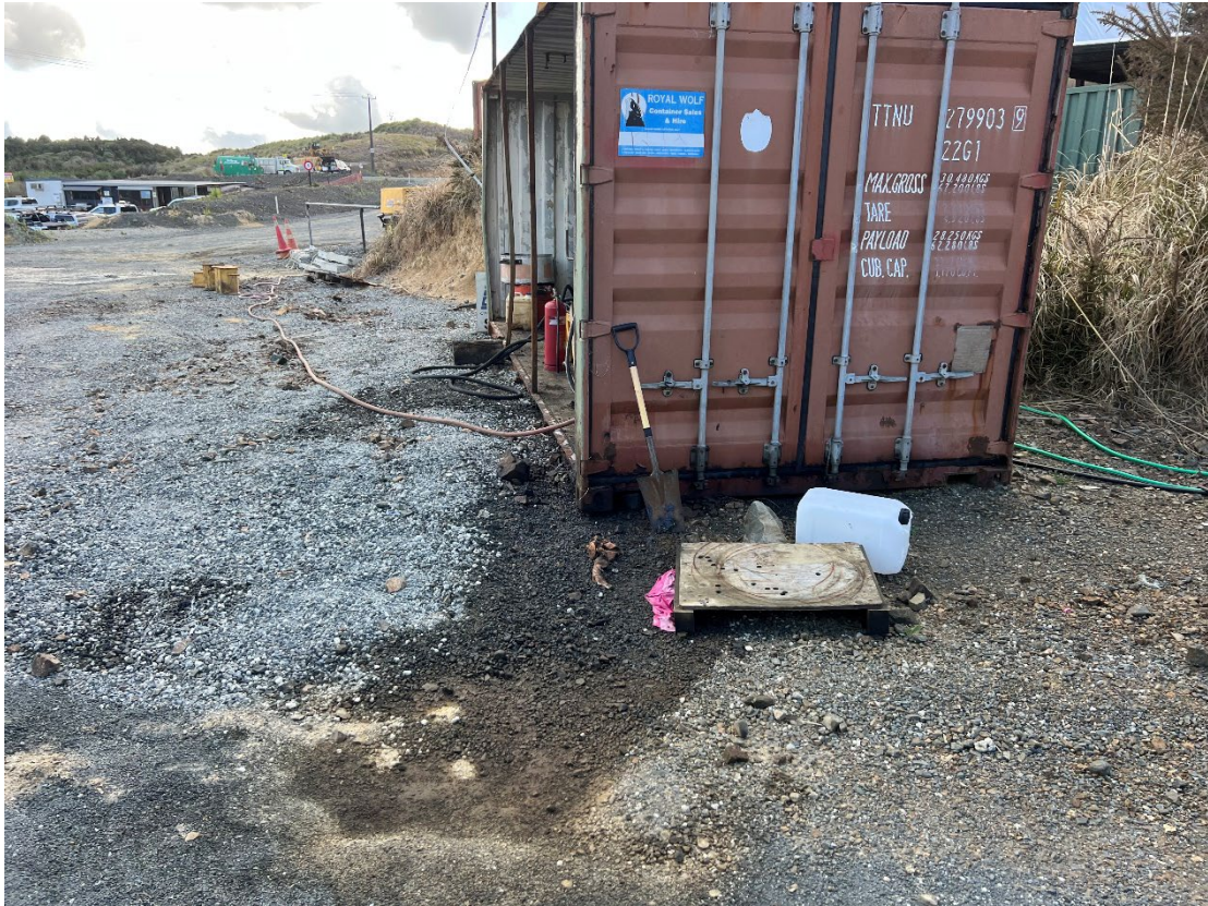
Photograph 15: Looking southeast at a shipping container (near the northwestern corner of the vehicle maintenance structure) where waste oil is temporarily stored with hydrocarbon staining on the ground where PMS16 was taken.
