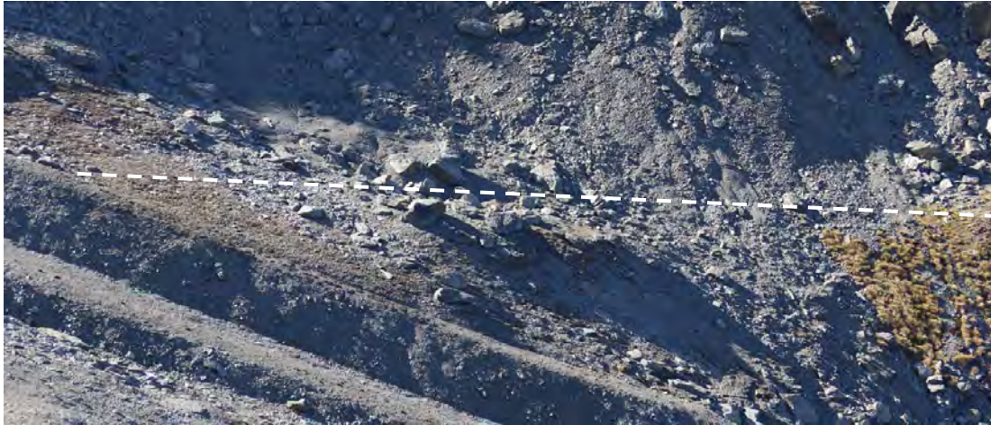
Figure 39. Debris field of large fallen rocks (and part of the unused half pipe) below the ridge line. Nominal route of proposed temporary access shown as broken line.
