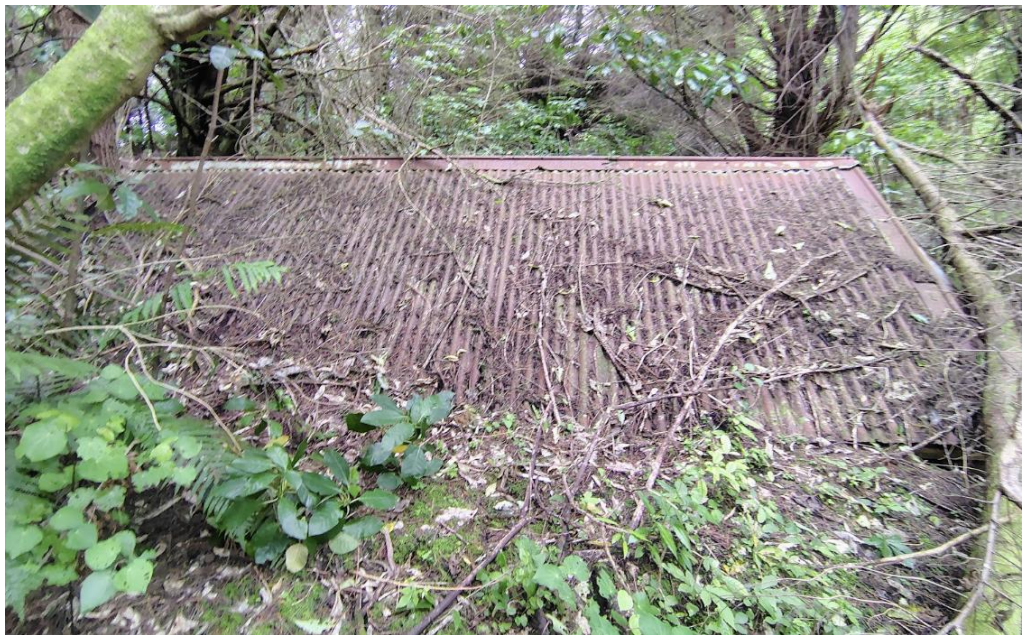
Figure 29. View of the corrugated metal roof of the collapsed farm building, looking east
