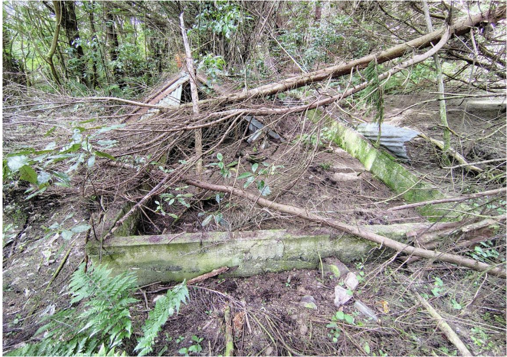
Figure 28. View of the collapsed farm building (R27/910), looking south
