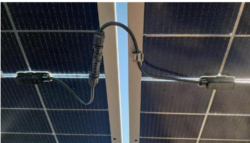
Figure 12: DC String cables (Source: HENZ – Tauhei Solar Farm)
