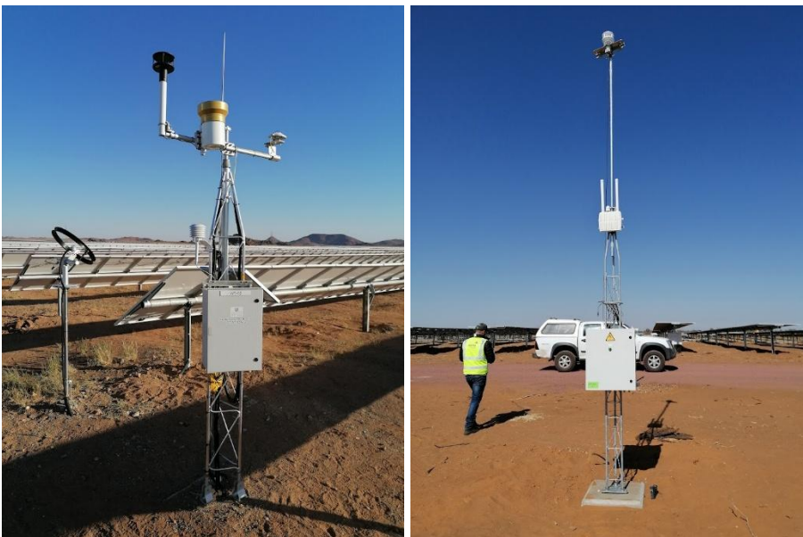
Figure 10: Example of a Meteorological Communication Unit
