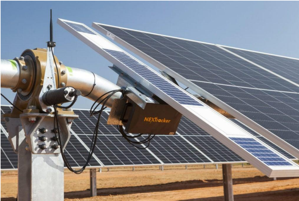
Figure 9: Tracker Self-Powered motor, solar module, battery and controller unit.. Source: https://www.pv-tech.org/nextracker-finalises-split-from-flex-and-becomes-independent-company/
