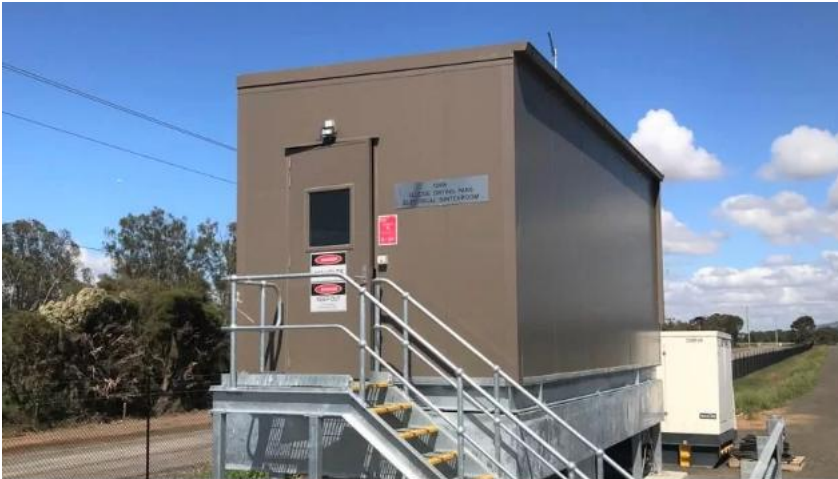
Figure 16: Switching Station (Example) Source: www.wibs.com.au/switch-rooms
