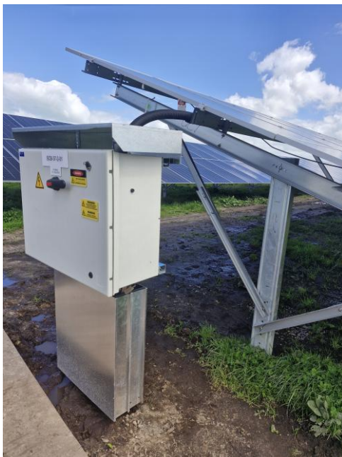
Figure 13: Example String Combiner Box (Tauhei Solar Farm)
