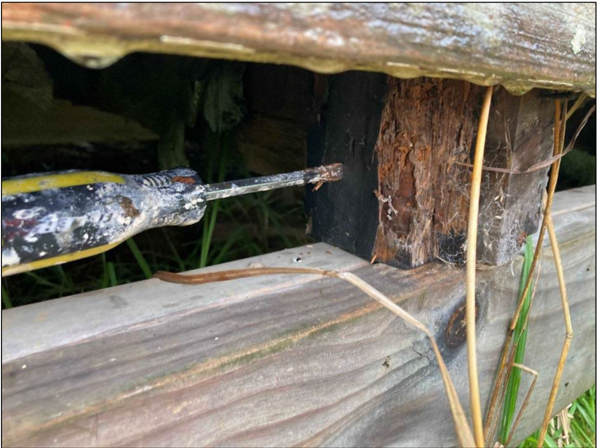
Figure 12. Blackened and decayed stud at the base of the east elevation.
