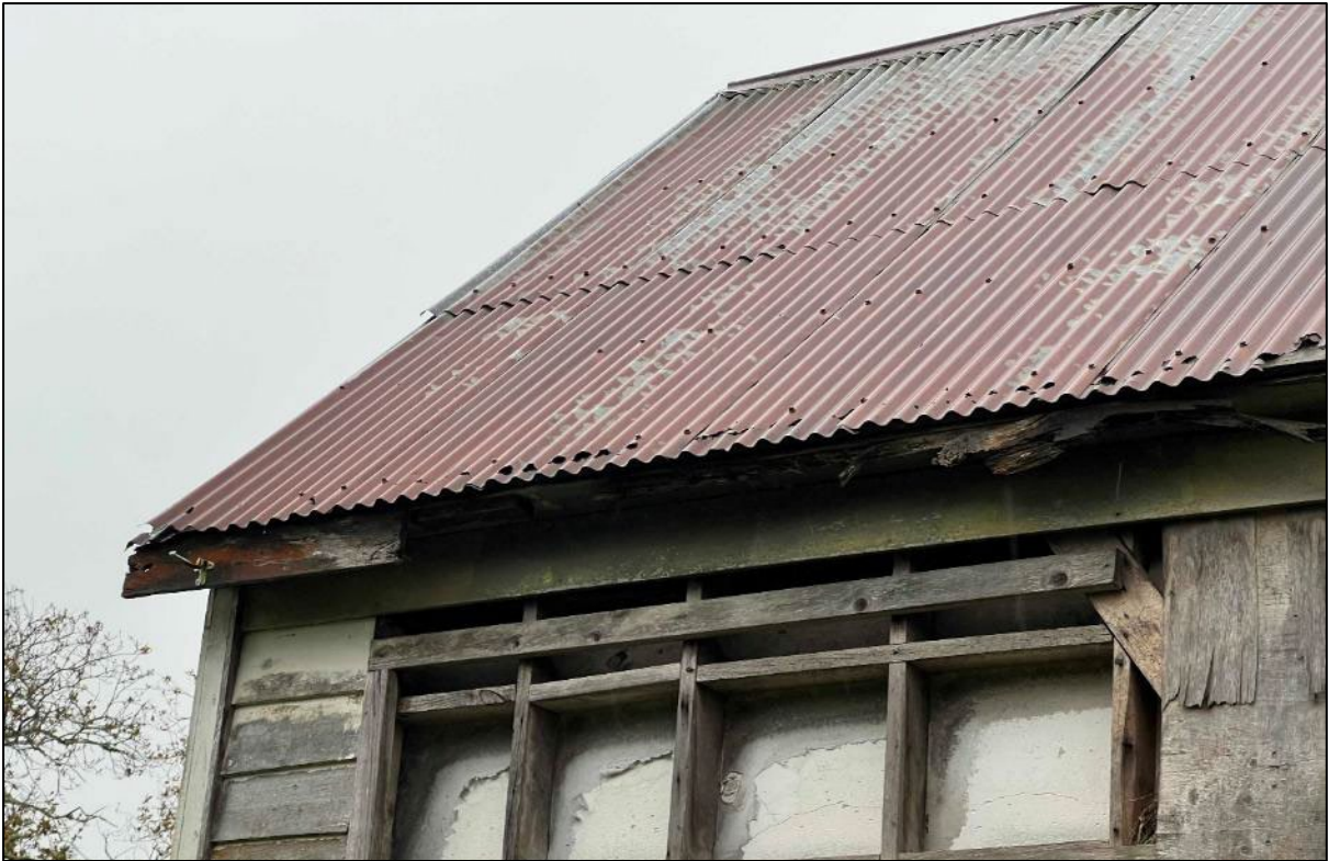
Figure 5. Eaves at the north-west corner. The holes in the roof sheet, decayed remnant of fascia, and single remaining gutter bracket are all evident.
