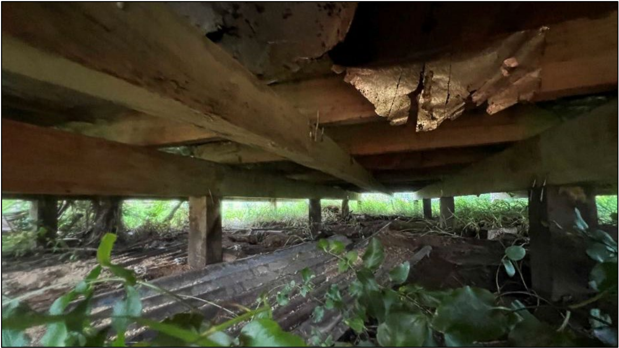
Figure 23. Subfloor: the c. 2010 bearers and piles fixed with stainless steel Z nails are visible on either side of the image. The member at the centre of the image is interpreted as relating to earlier renovations and is fixed with galvanised Z nails.
