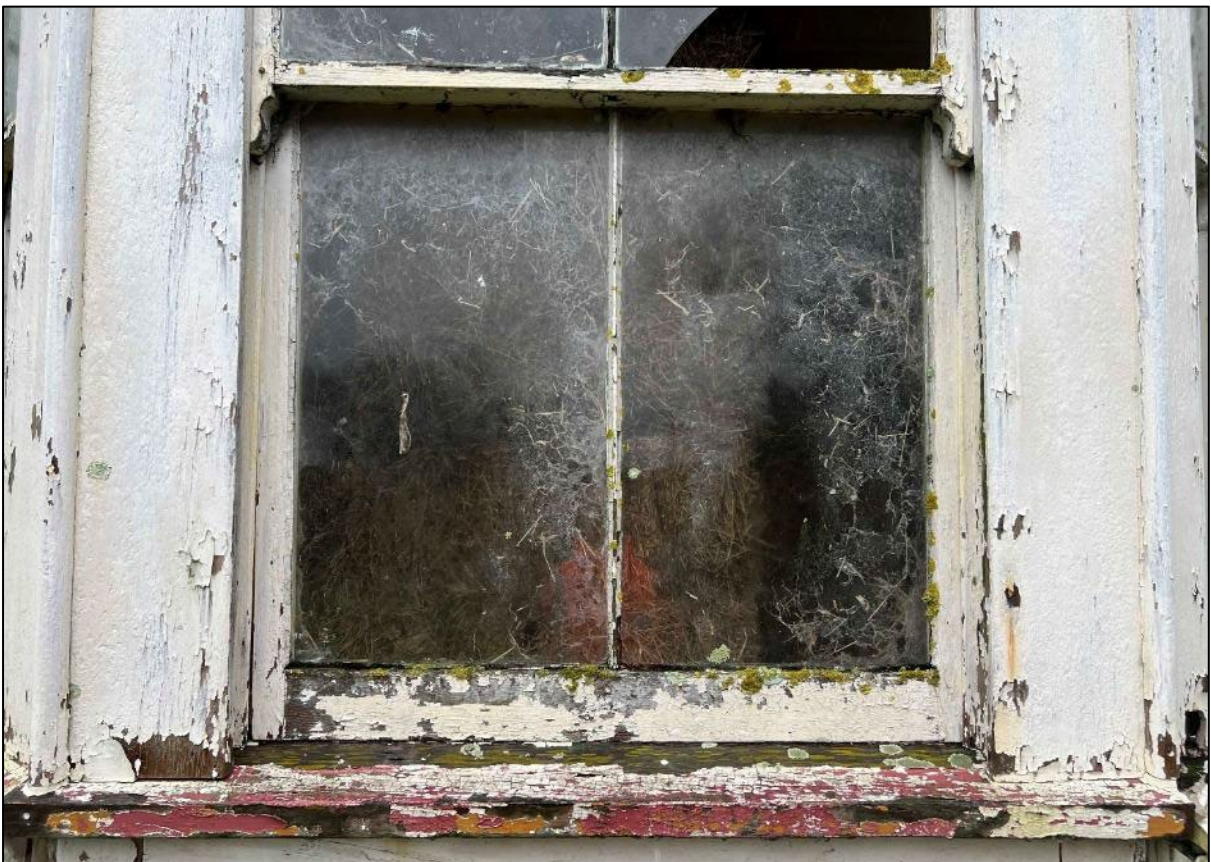
Figure 16. Detail of lower sash of the central part of the bay. Note the broken pane in the upper sash and missing putty.
