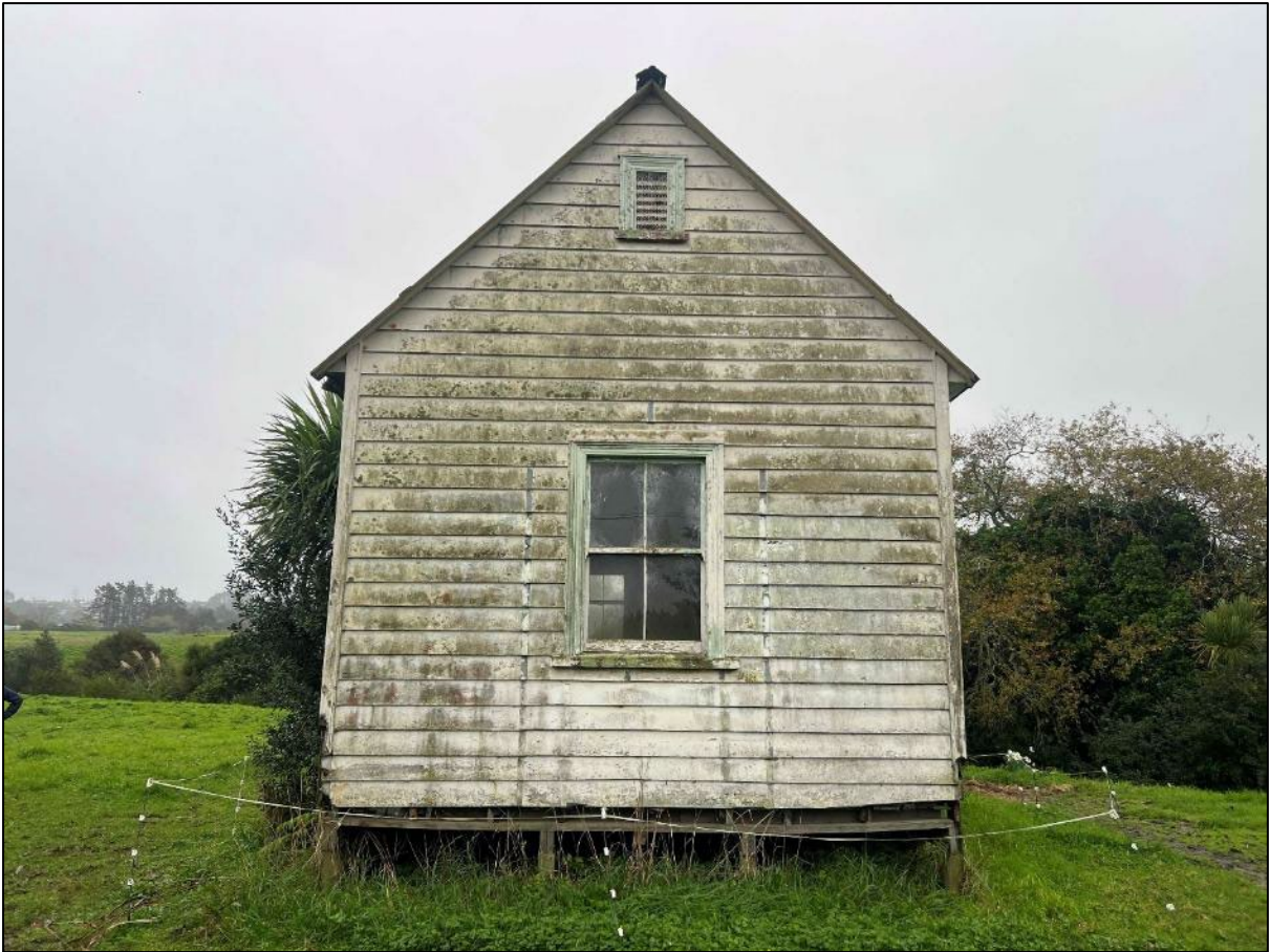
Figure 9. South elevation. Note the steel strips visible over joins in weatherboards and the bowed baseplate.
