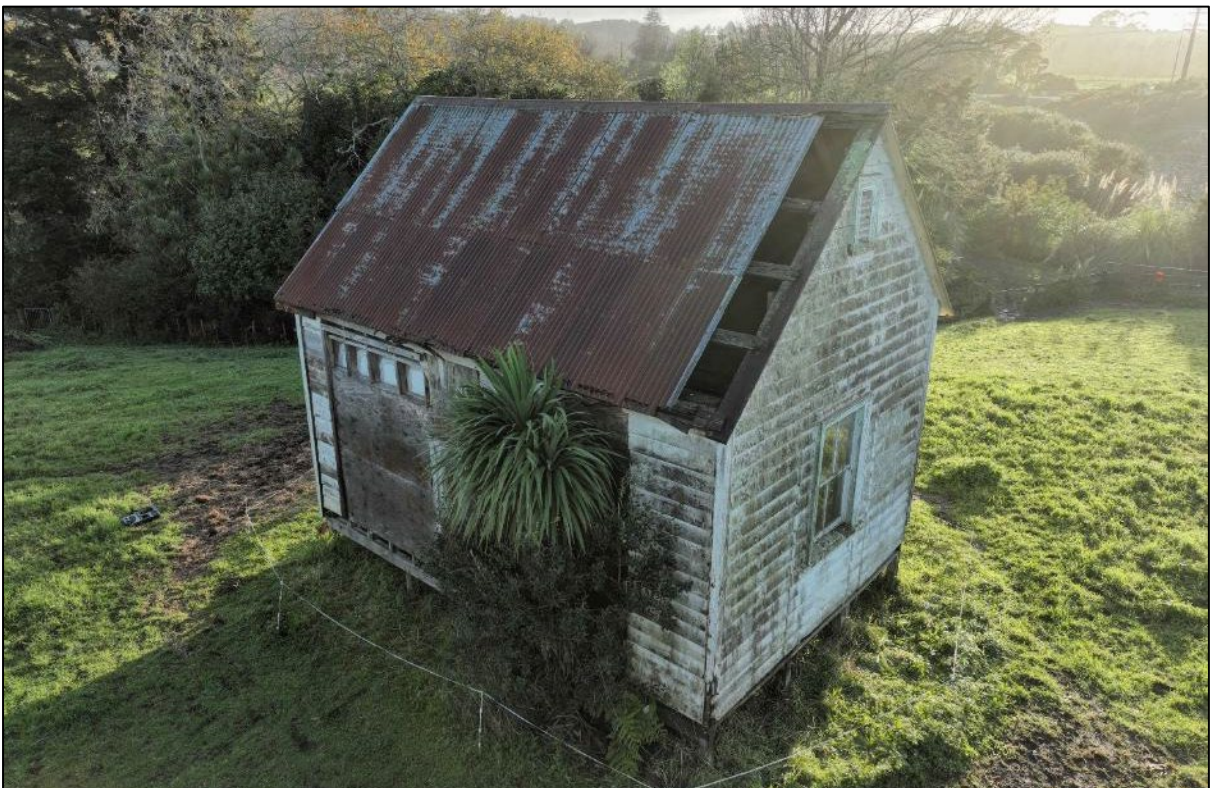
Figure 4. West and south elevations of the meeting house showing the corroded roofing and missing sheet.
