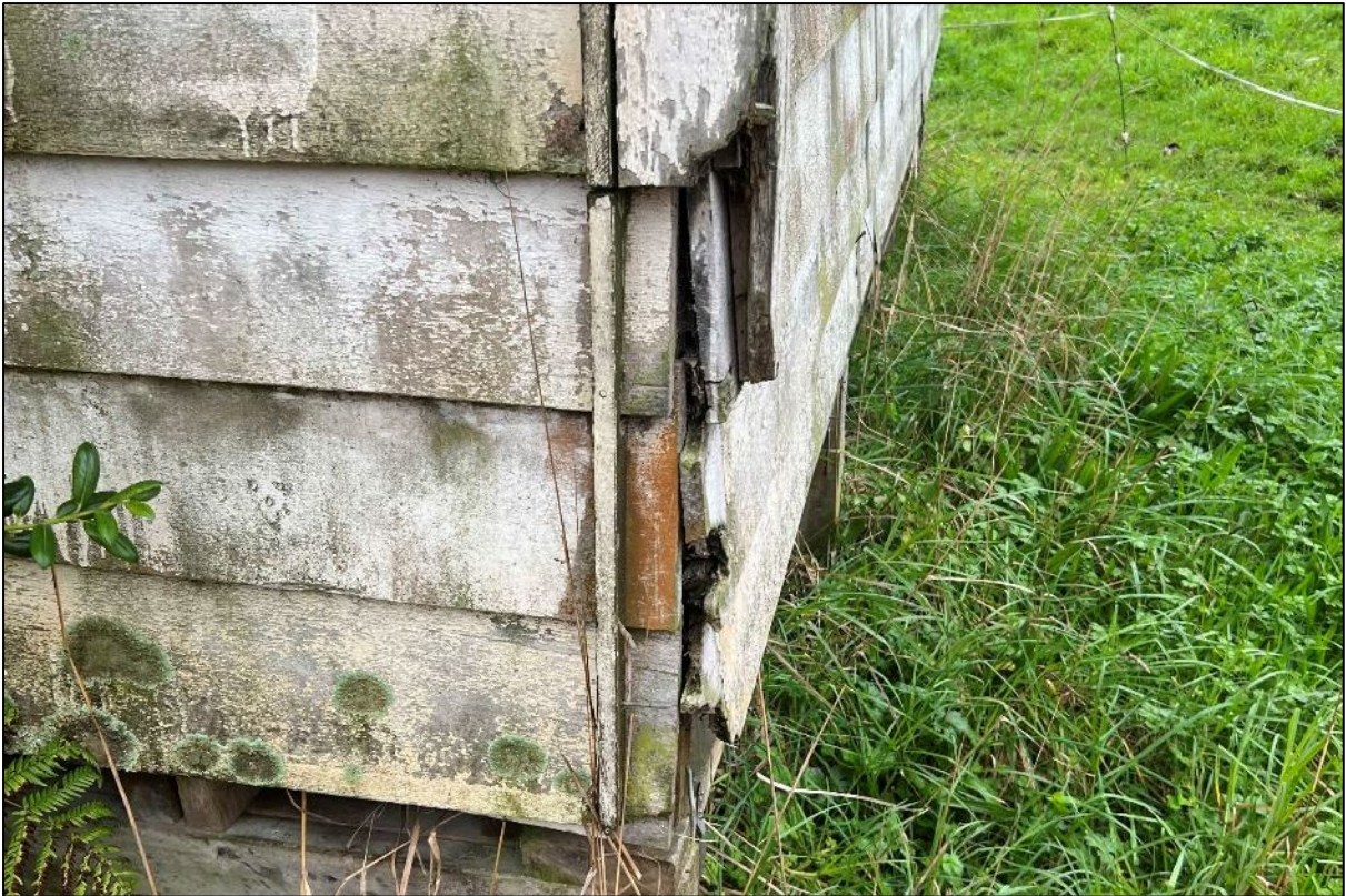
Figure 11. Decayed boxing at south-west corner.
