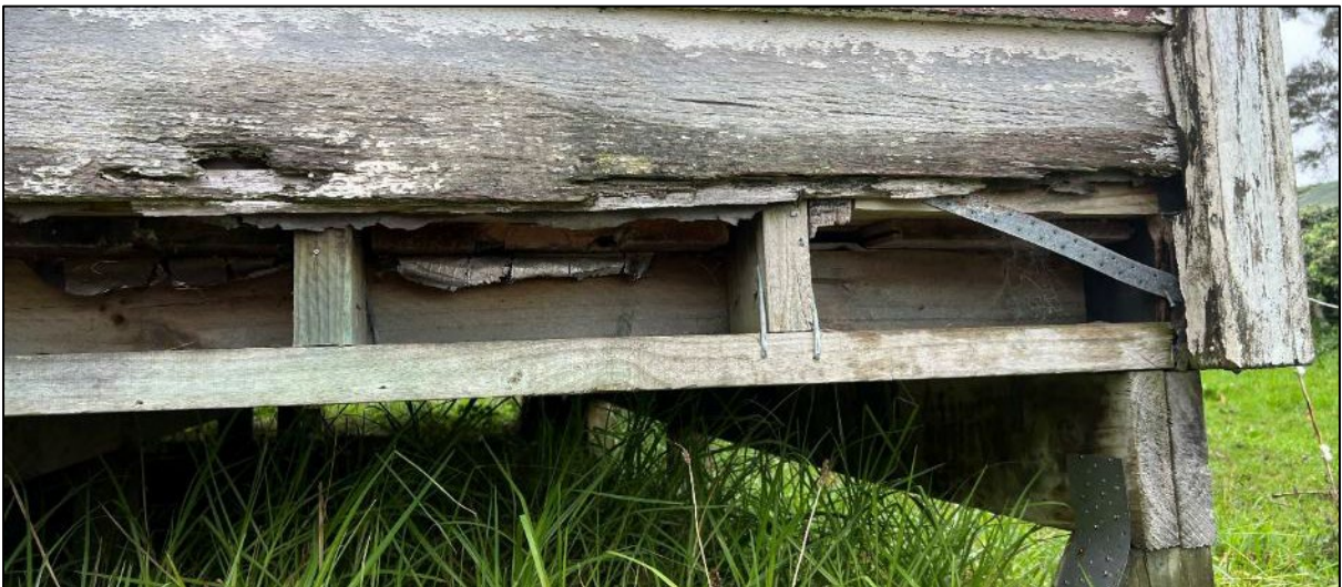
Figure 8. Decayed weatherboards on the north elevation.
