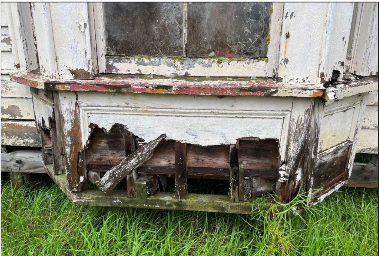
Figure 14. Decayed cladding at the base of the east elevation bay window.
