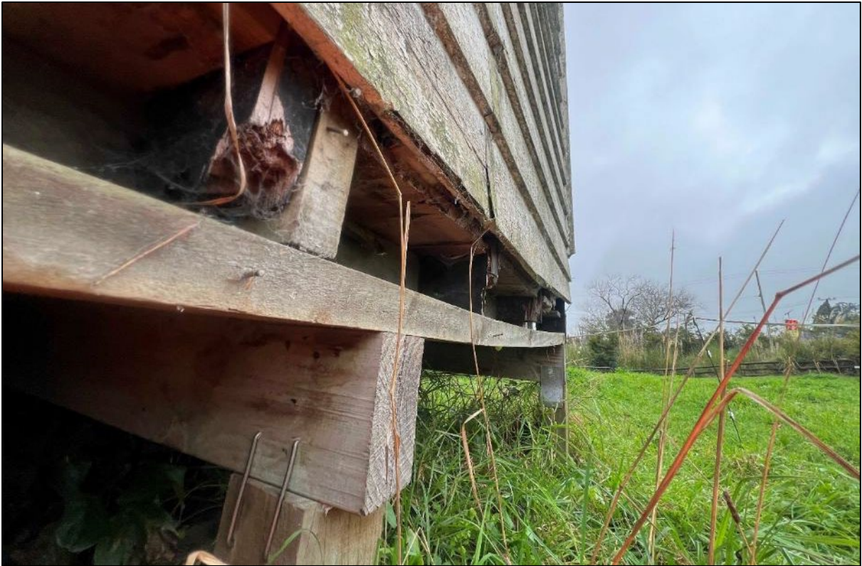
Figure 13. Bowed bottom plate on south elevation, looking east.
