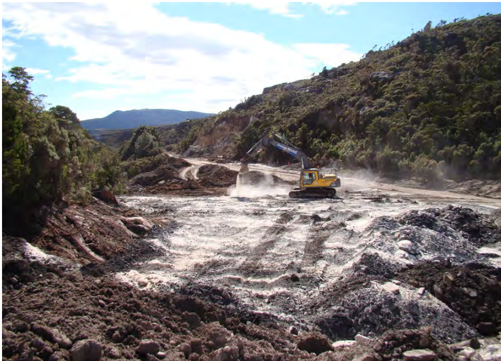
Figure 45. Limestone dosing of the BV ELF.
