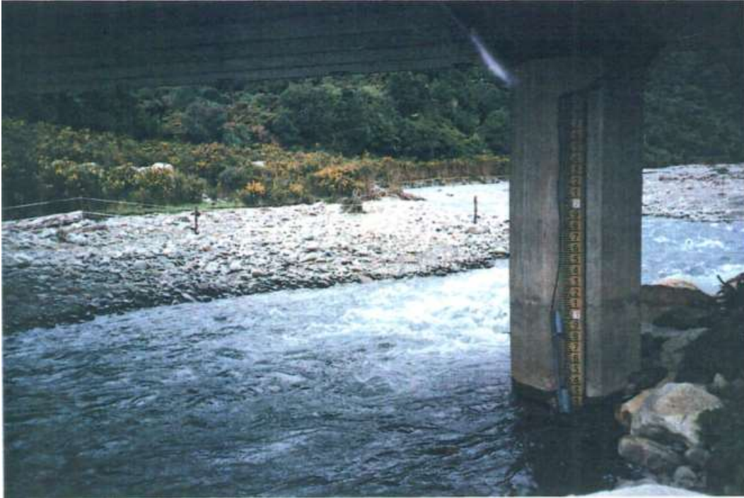
Figure 40: 1990s-era Canoe Creek hydrological site at SH6 bridge pylon, including sight board and river stage sensor cables (Coffey & Partners, 1991)
