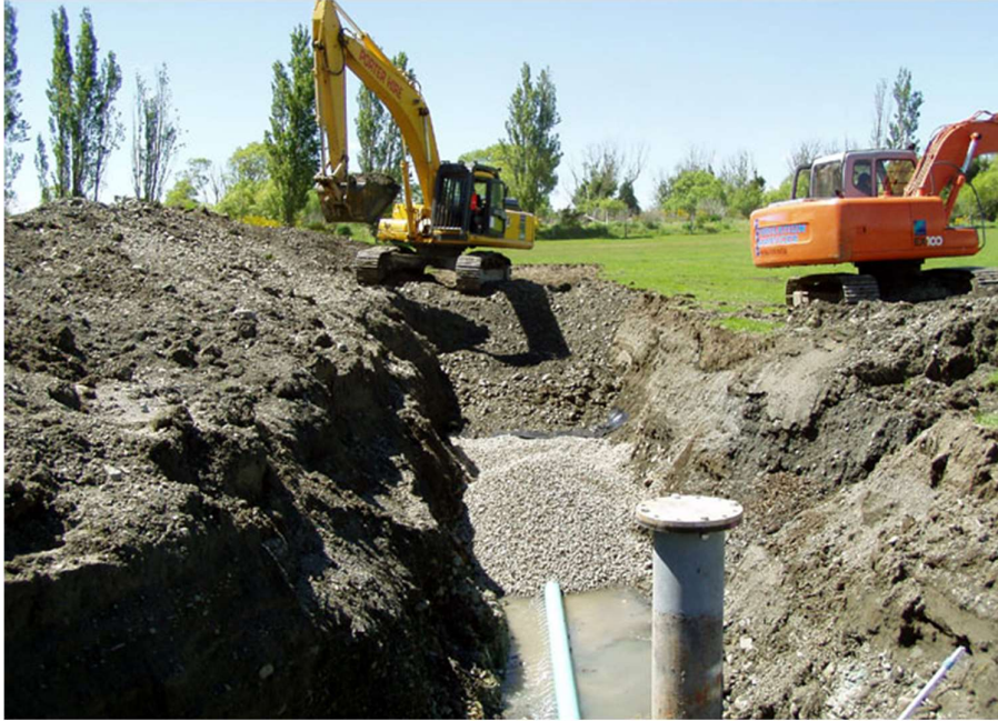
Figure 32: Example of infiltration gallery construction [photo credits to Butt Drilling Ltd (buttdrilling.co.nz)]
