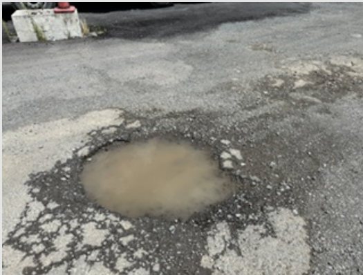
Pothole in Les Harrison Transport Yard
