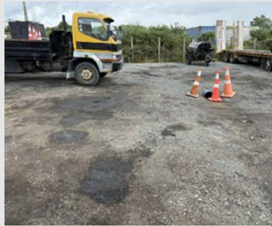
Hydrocarbon staining in storage yards
