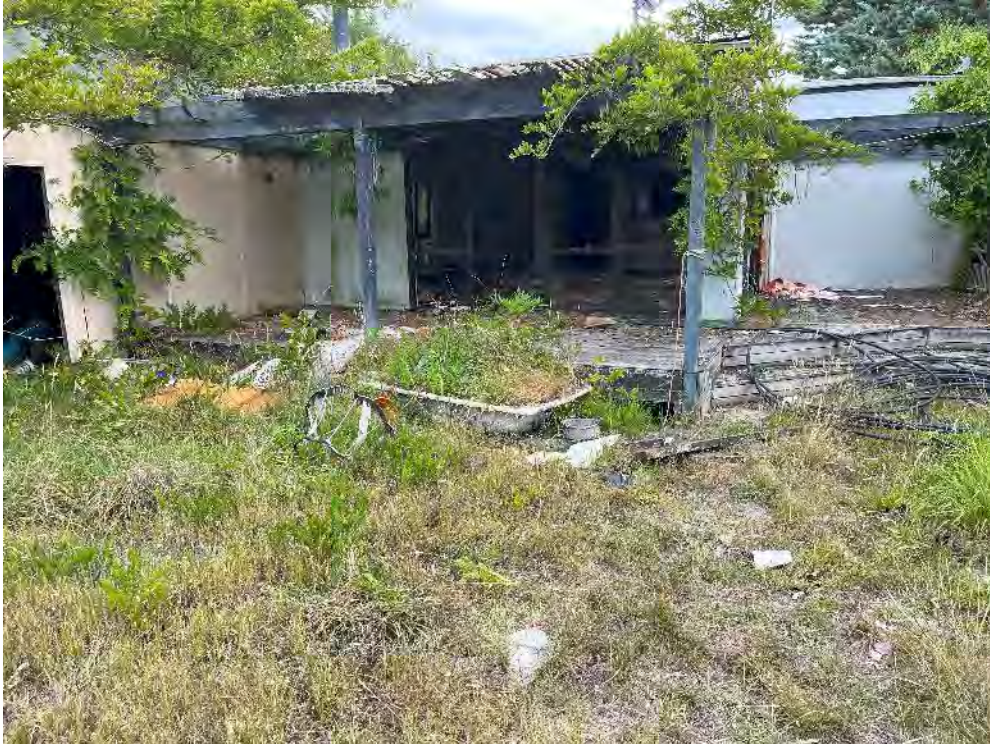
PLATE 5: Dwelling 5 with fragments of suspected ACM within the yard in the foreground.
