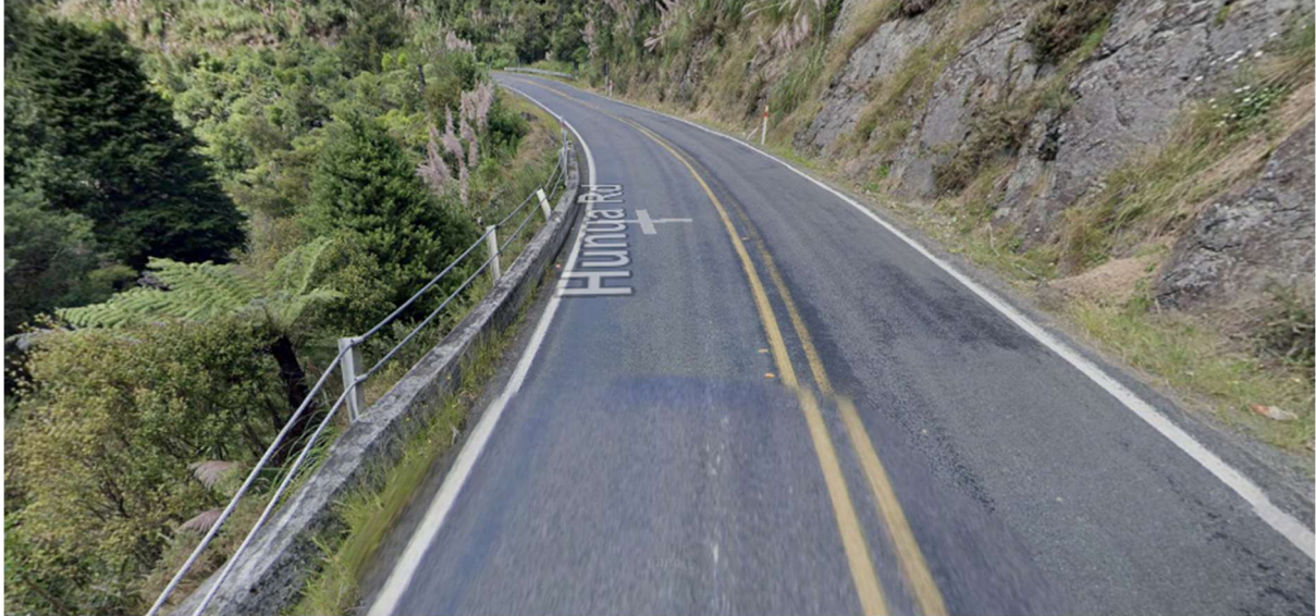
Photo 3: Road safety barrier next to gorge on Hunua Road. Corresponding Commute tracking drawing number 4D.
