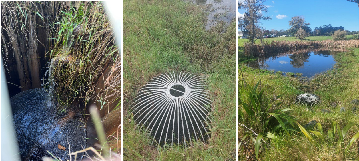
Photo 2: Scruffy dome draining Pond 2.
