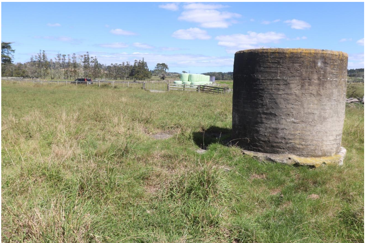
Figure 87. View facing southwest showing the overgrown slab and relocated water tank
