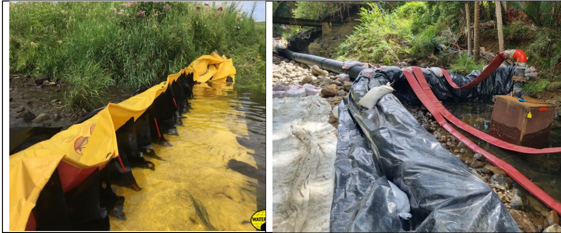
Figure 24: Example of a hydro barrier (left) and sand bag coffer dam (right) iii
