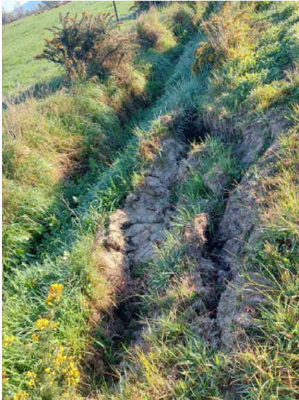
Figure 5. Whites Road drain condition, 29 September 2026 showing major slumping.
