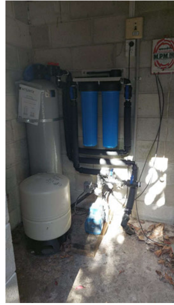
Figure 10: [REDACTED] filtration system installation required following water test results September 2026.
