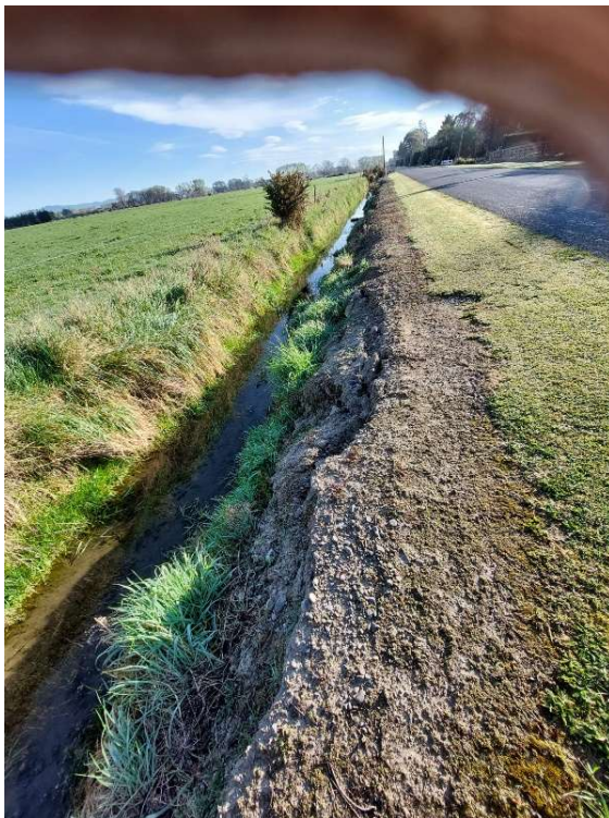
Figure 7. Whites Road drain condition, 29 September 2026.
