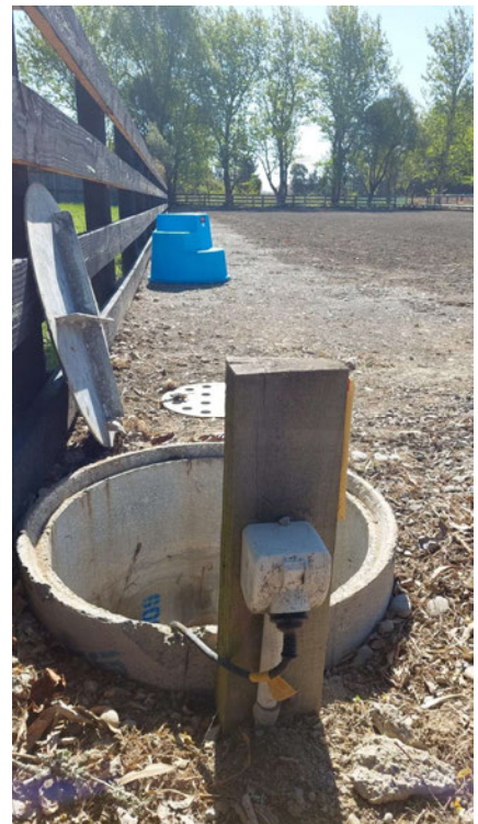
Figure 8. Sump and pumping station installed to manage surface-water runoff at [redacted] after 2022 flooding that entered sleepout and workshop.
