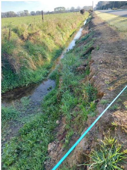
Figure 1. Whites Road drain condition, 29 September 2026, showing unstable, crumbling, sloping edges from narrow verge.
