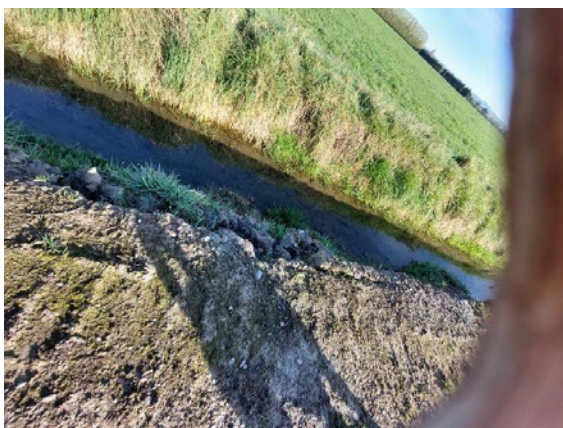
Figure 3. Whites Road drain condition, 29 September 2026, showing unstable edges
