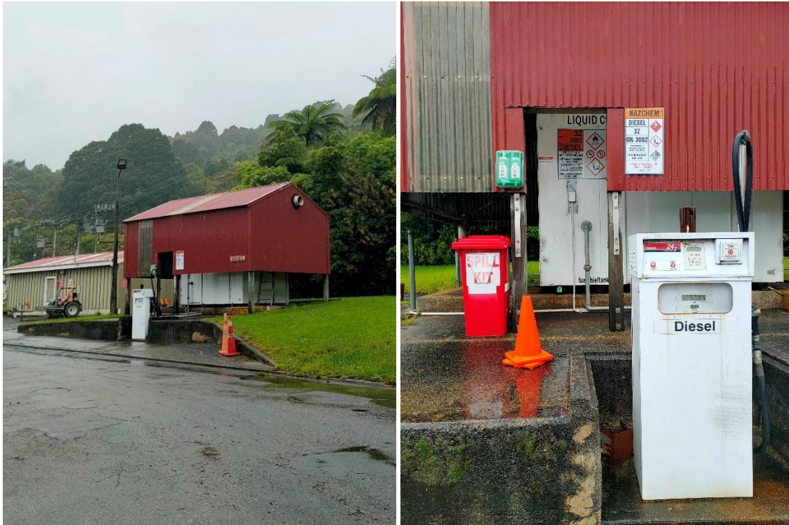
Figure 6.3: Covered diesel tank and fuel dispenser (left), close up of fuel dispenser (right).
