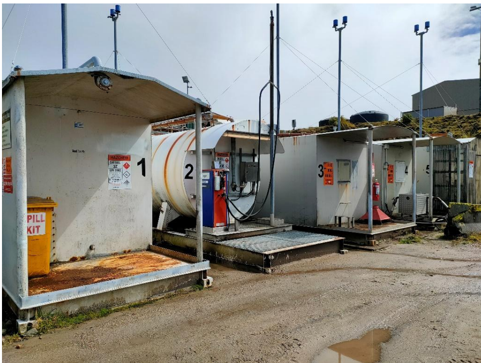
Figure 6.5: Bulk diesel tanks (right).
