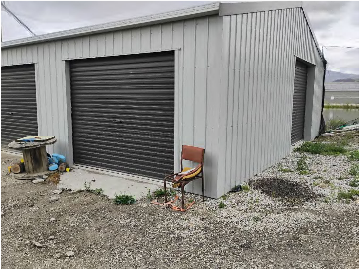
Figure 37: Minor patch of oil staining.
