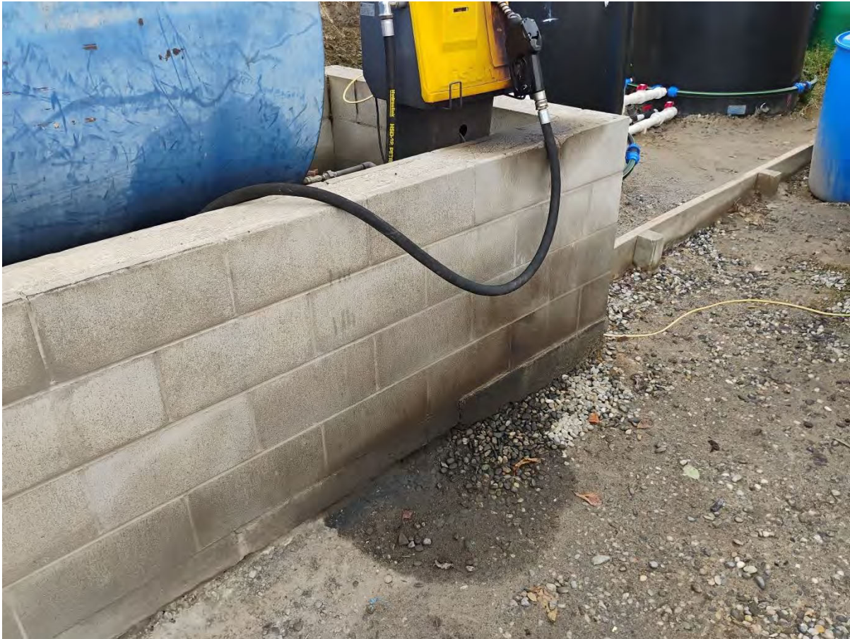
Figure 23: Minor staining beneath the diesel dispenser.
