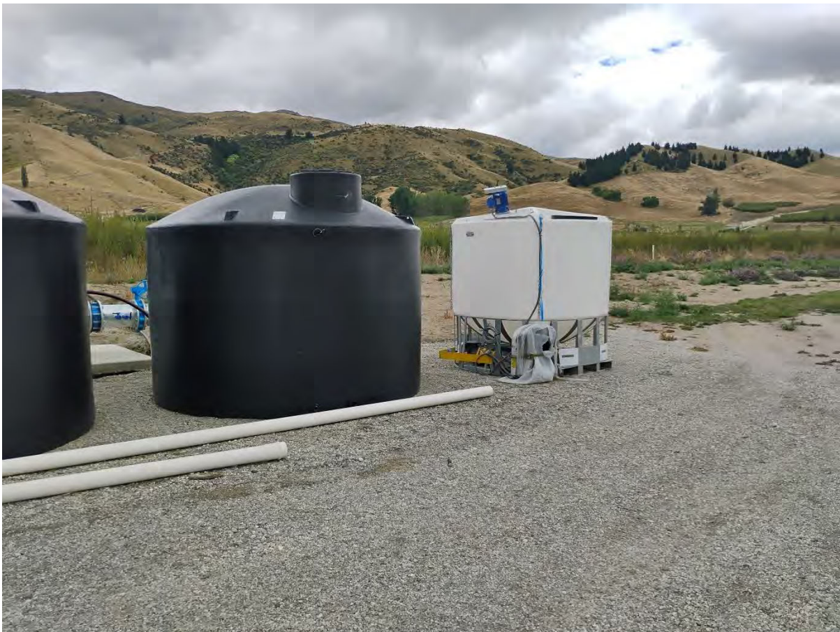
Figure 2: Storage tanks near the new pump shed on the western boundary of the site
