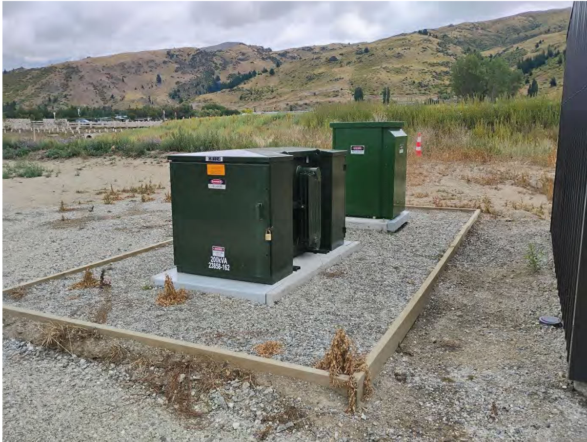
Figure 3: New transformers near the pump shed on the western boundary of the site.
