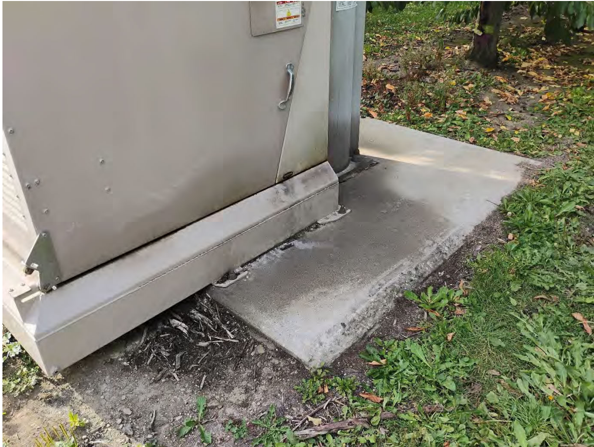
Figure 17: Minor lubricating oil staining on concrete
