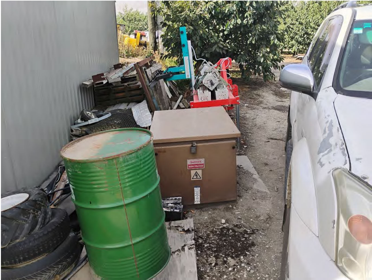
Figure 27: Transformer next to workshop building
