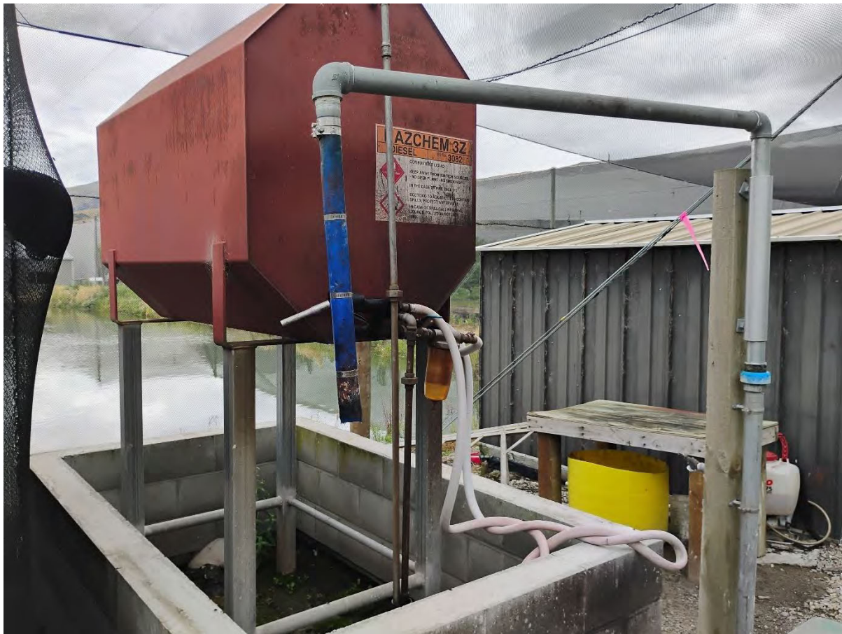
Figure 32: Above ground diesel tank
